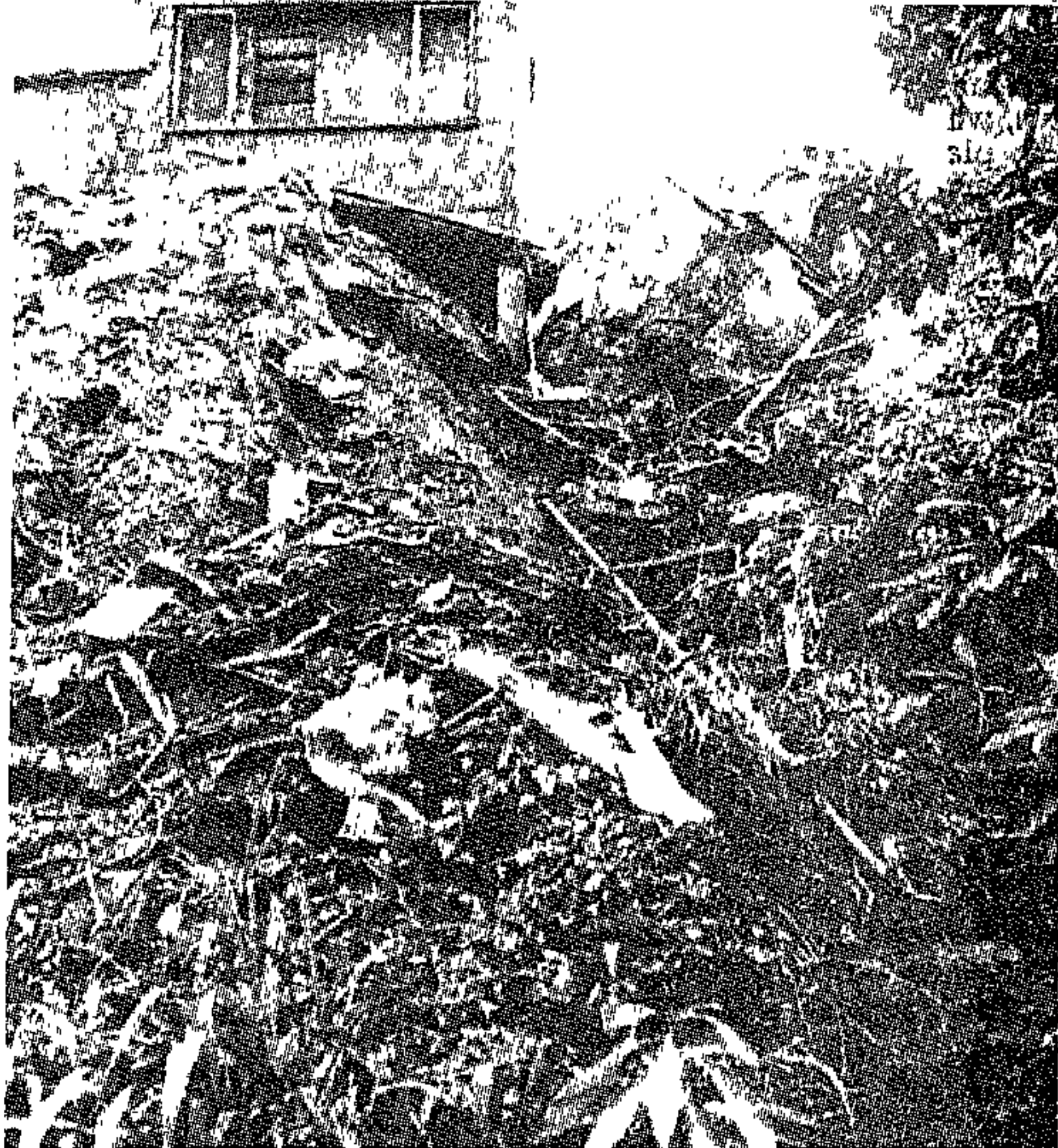
MUD FALL: The foundations of this building were undermined in the deluge which hit Durban on Saturday.
