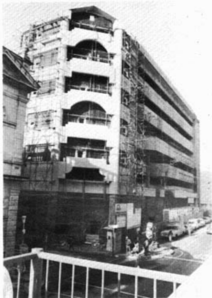
THE Murray and Roberts site in Cape Town where the workers went on strike recently.
