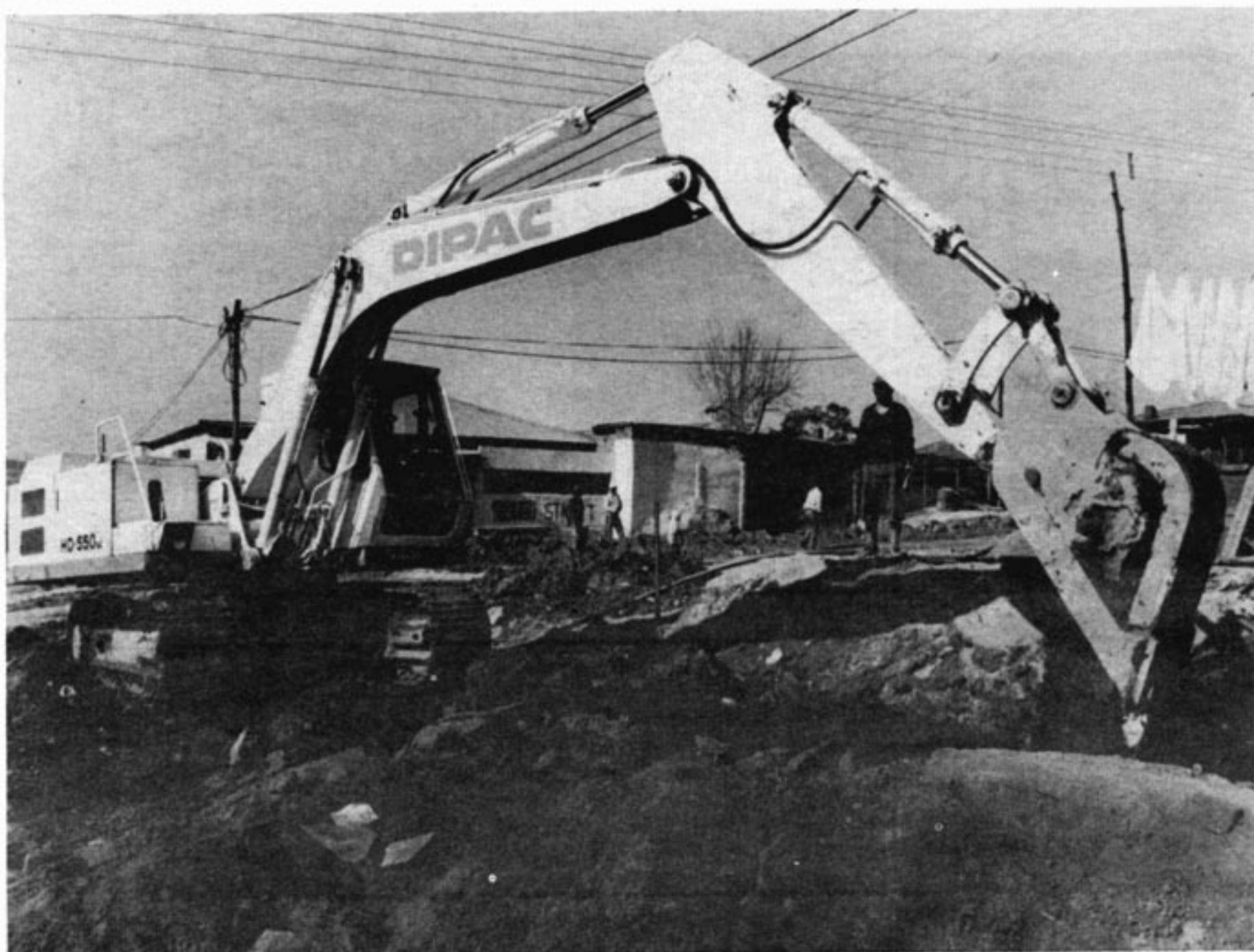
A construction company busy upgrading an African township: new pavements and a couple of tarred roads have never yet bought a people's soul
