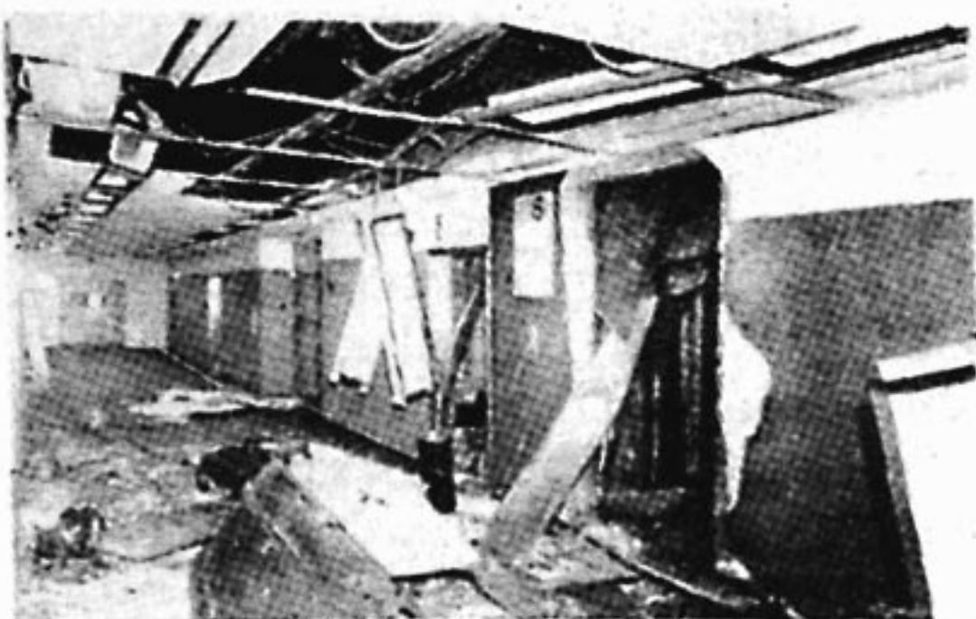
The badly damaged sixth floor of the 'Presidential Council' building.
