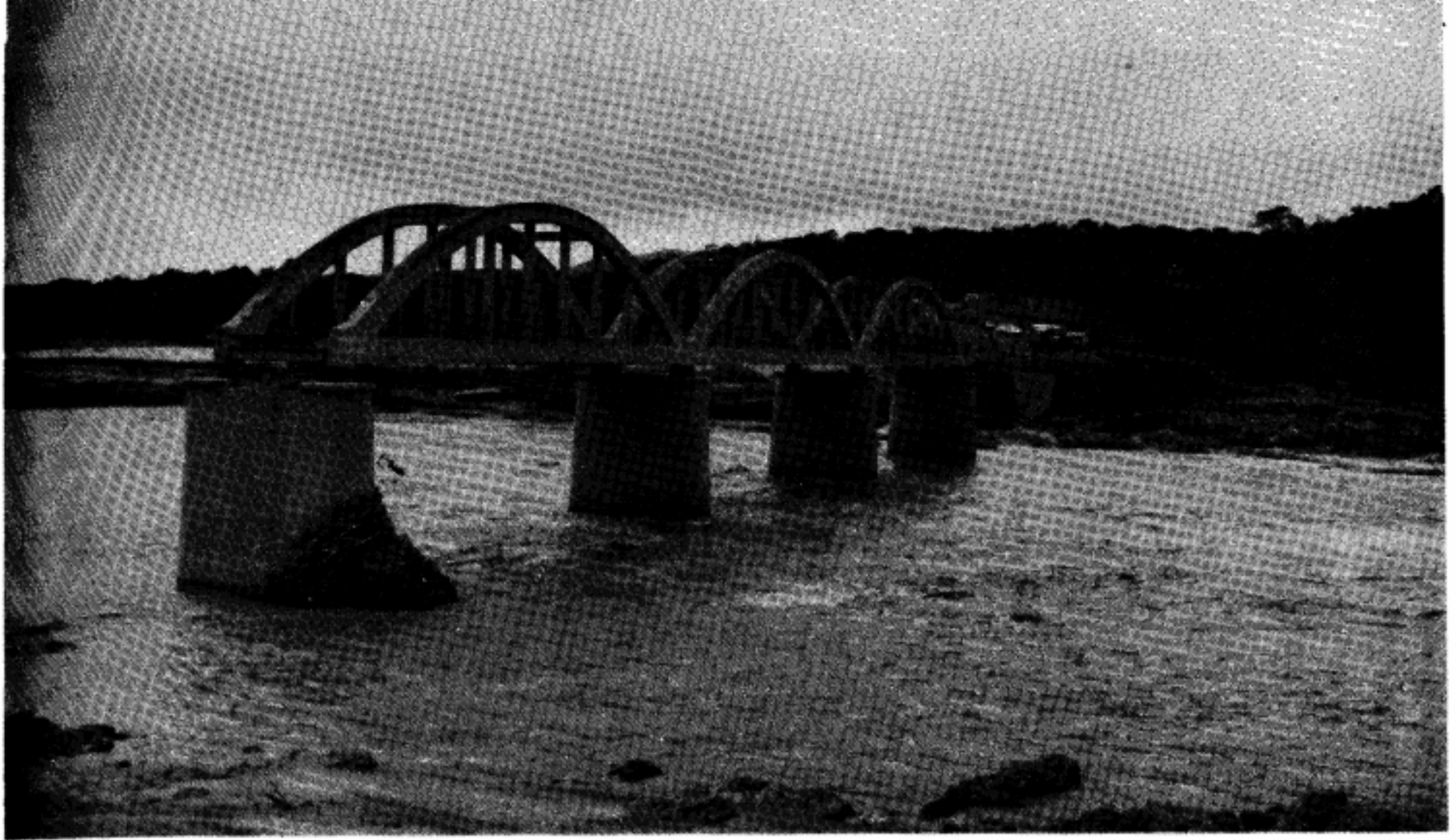
White Umfolozi Bridge — broken
