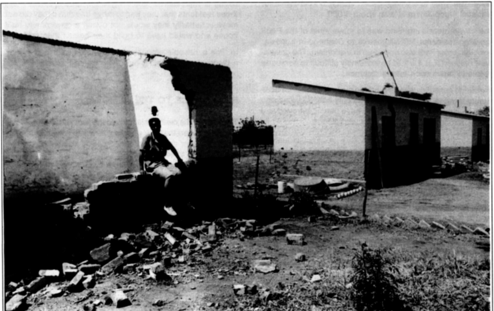
Wanton destruction of housing in Tshikota
