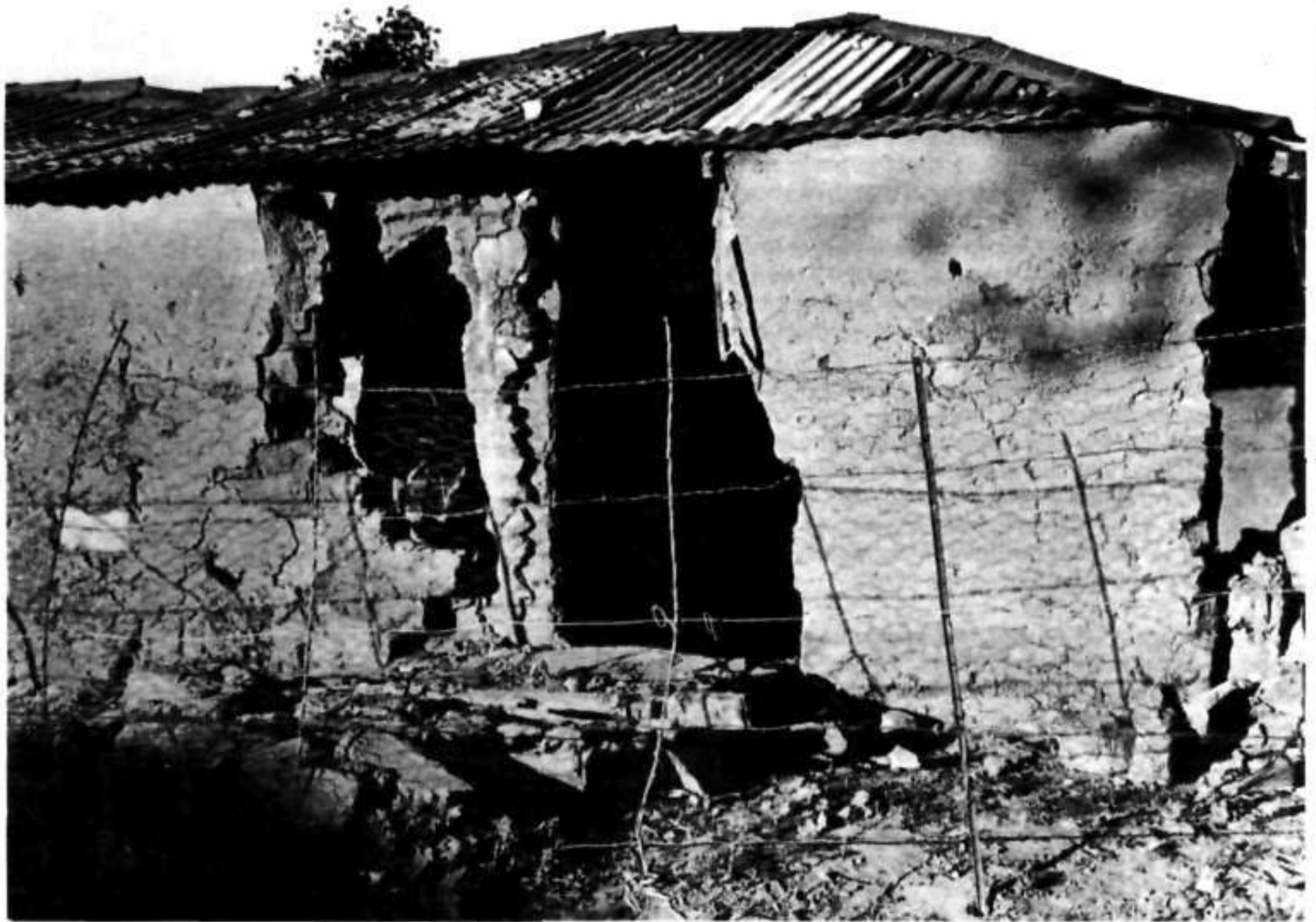
Huhudi — a decaying home. Residents were not allowed to renovate for many years
