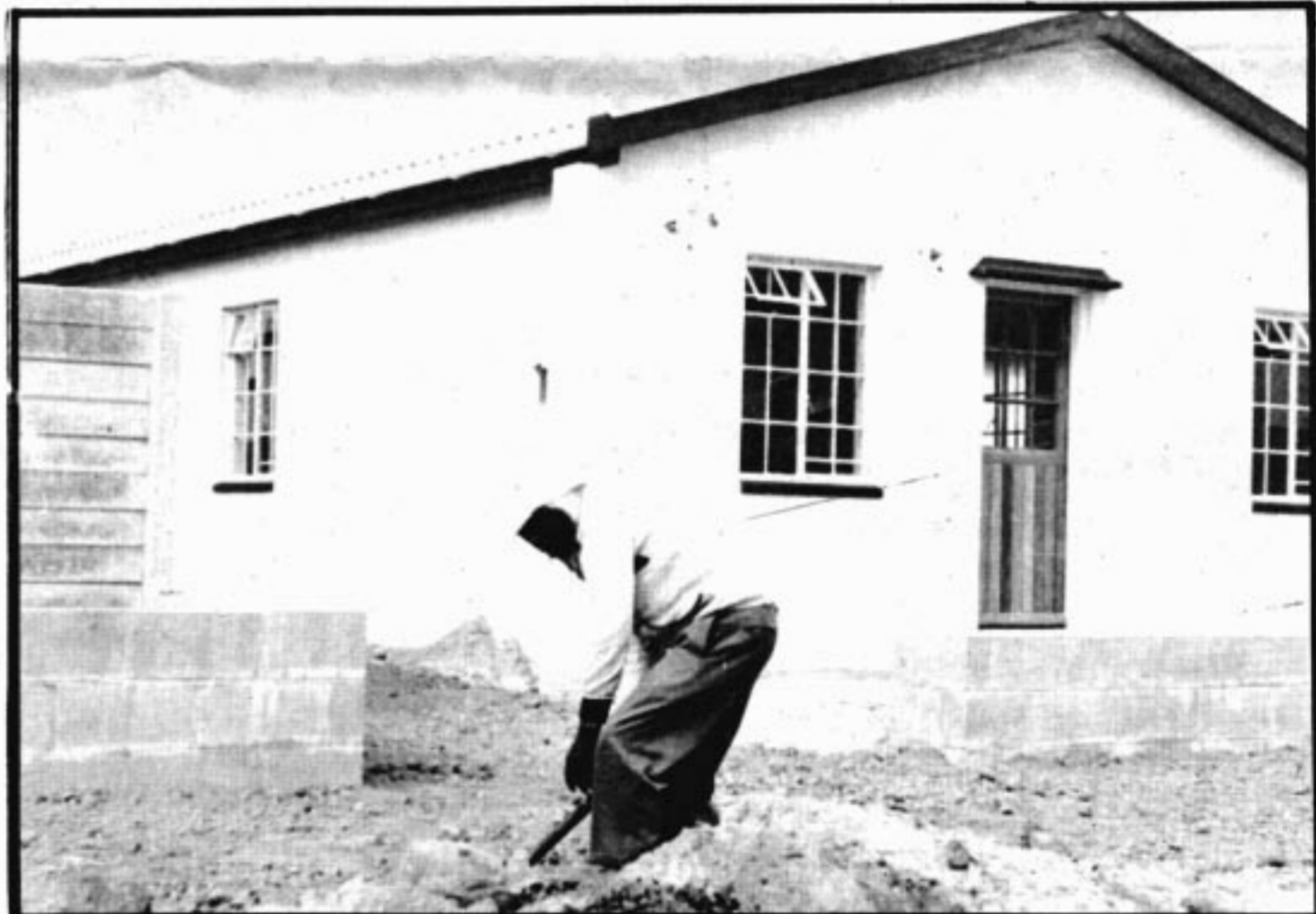
A worker outside one of the 'instant houses' in New Tafelsig Area
