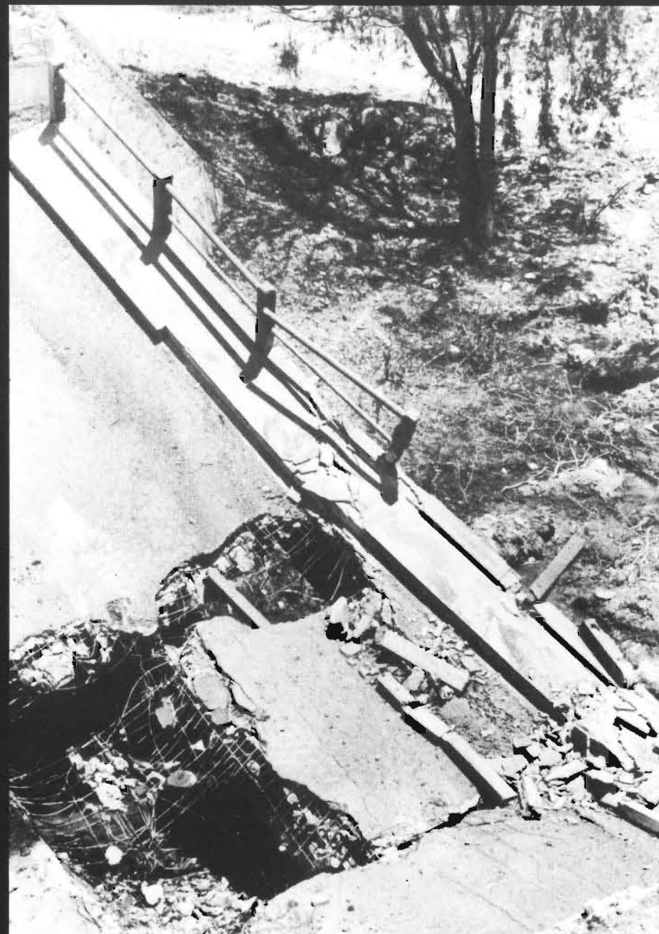
▲ Angolan road bridge destroyed by South African bombing
