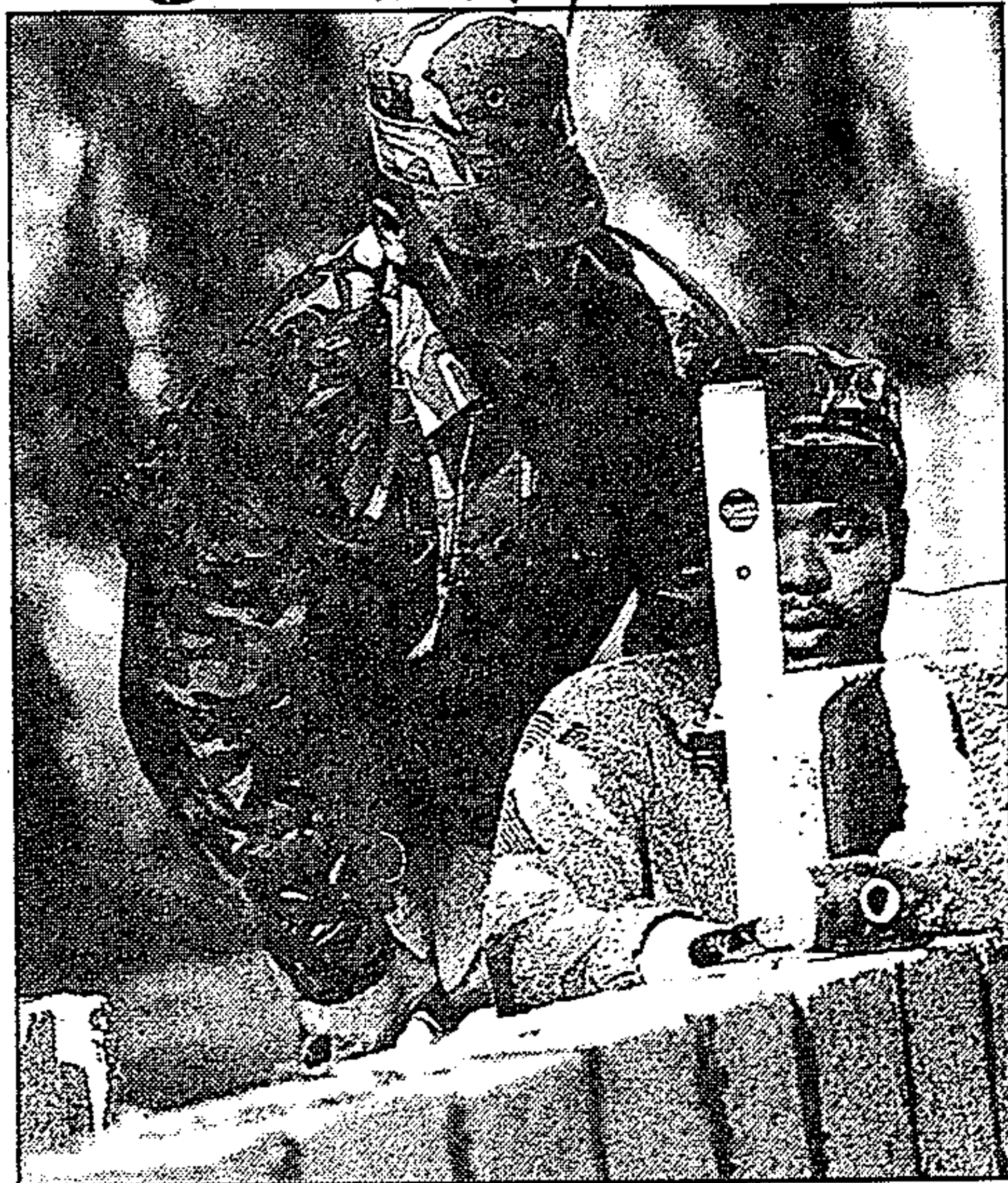
Laying foundations . . . ex-MK cadres work at the Shaft 17 training centre in Crown Mines. PICTURE: RUVAN BOSHOFF
