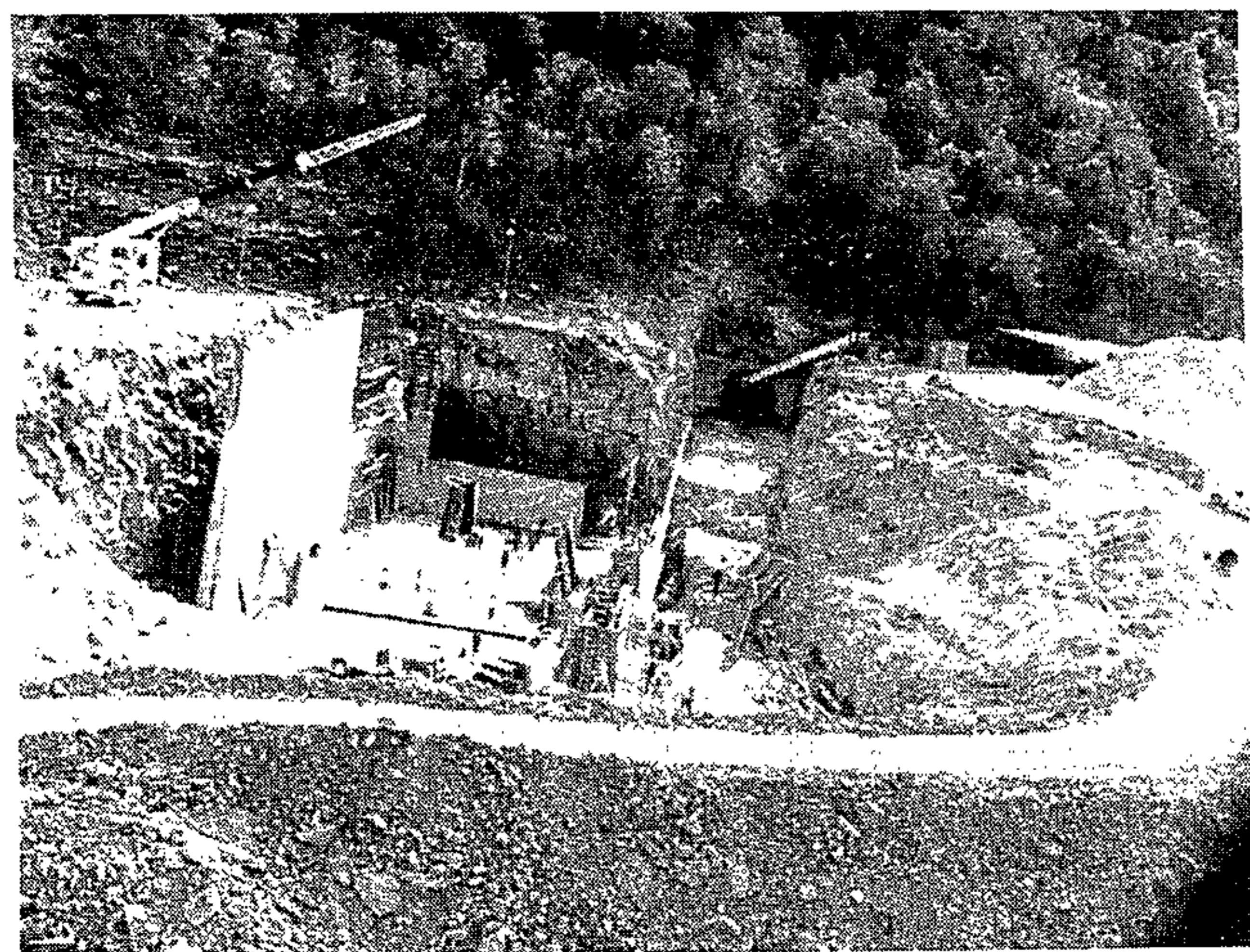
MBASHEE HYDRO ELECTRIC STATION UNDER CONSTRUCTION ● POWER STATION BUILDING AND TUNNEL OUTLET
