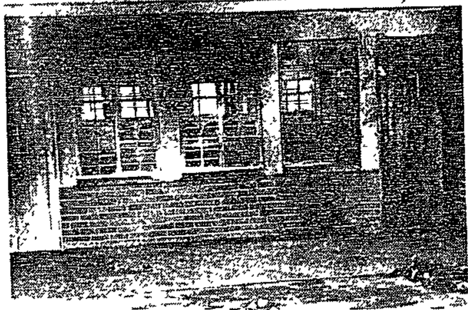
A section of the Zone One rent office in Mdantsane which was damaged by fire and stoned early yesterday.
