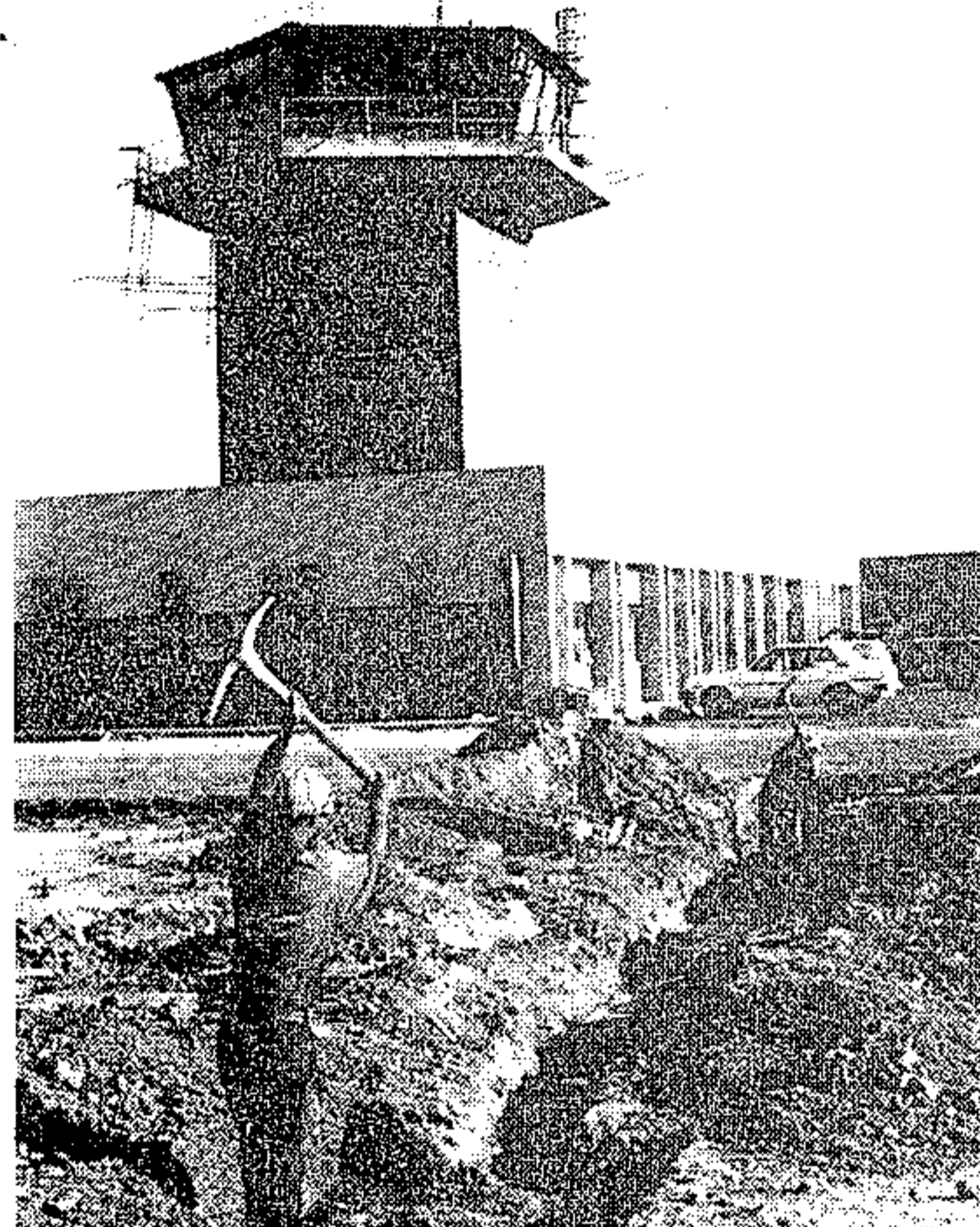
The deserted control tower. In two months it will be a hub of activity as traffic controllers keep a sharp eye for approaching and departing aircraft.
