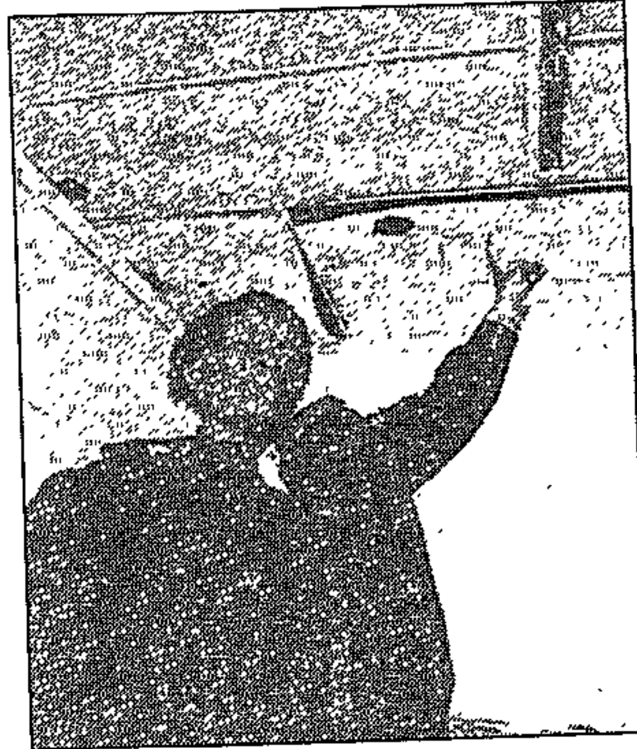
Matron Rosebelle Jele points to a dilapidated ceiling in a kitchen at St Lucy's Hospital. PIC: LEN KUMALO
