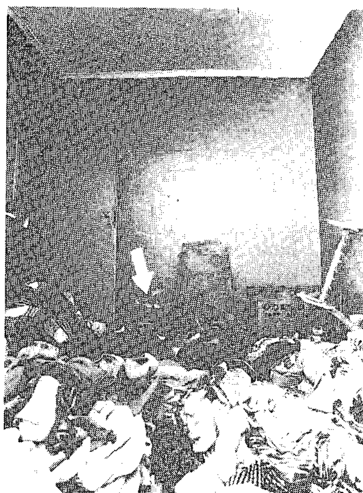
Arrows show where bullets penetrated the wall in yesterday's shootout.
