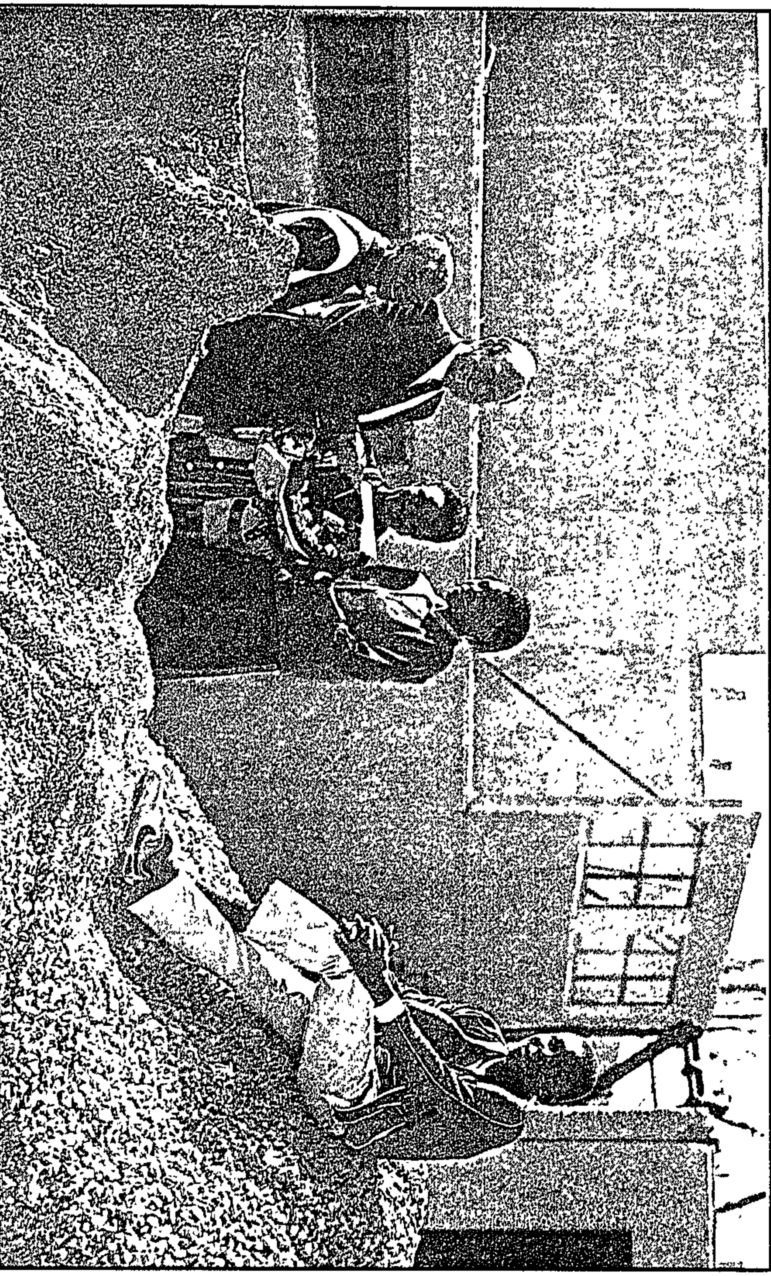
Happiness is seeing the walls of the technical college you hope to attend one day rising around you. Four youngsters, Violet Masuku, left, Priscilla Hlongwane, Santha Masilela and Simon Fabatsa, were on site at the new ACE College in Alexandra when Alan Tindall, chairman of the Allied Educational Trust, handed over a cheque for R50 000 towards the project. ACE steering committee chairman, Jolyon Nuttall, general manager of The Star, noted that R4,4 million of the R5,5 million needed had now been raised.
