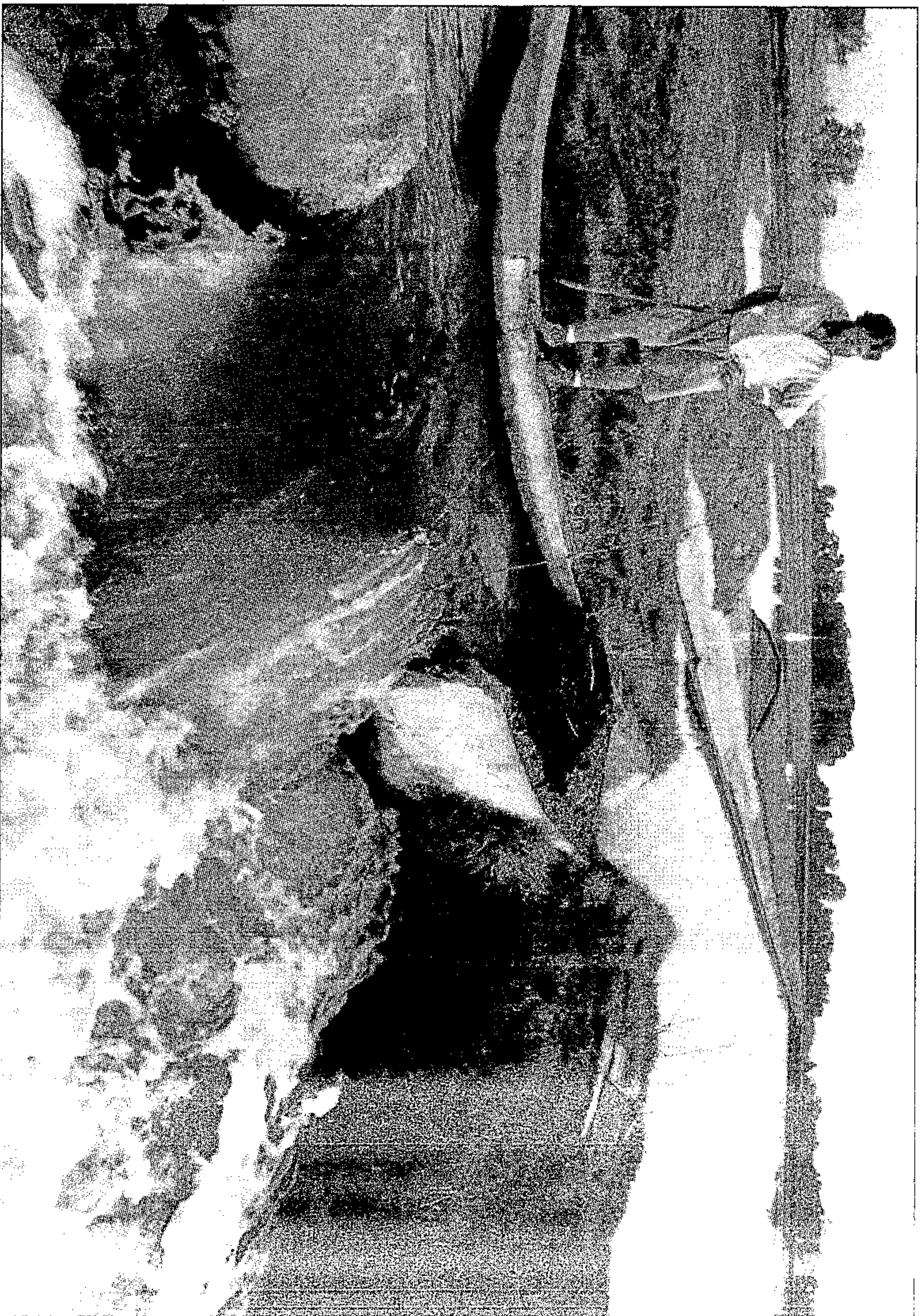
DIVERTED: A broken wall diverts polluted effluent from the maturation plant into which it should be flowing and allows it to tumble directly into the Klip River
