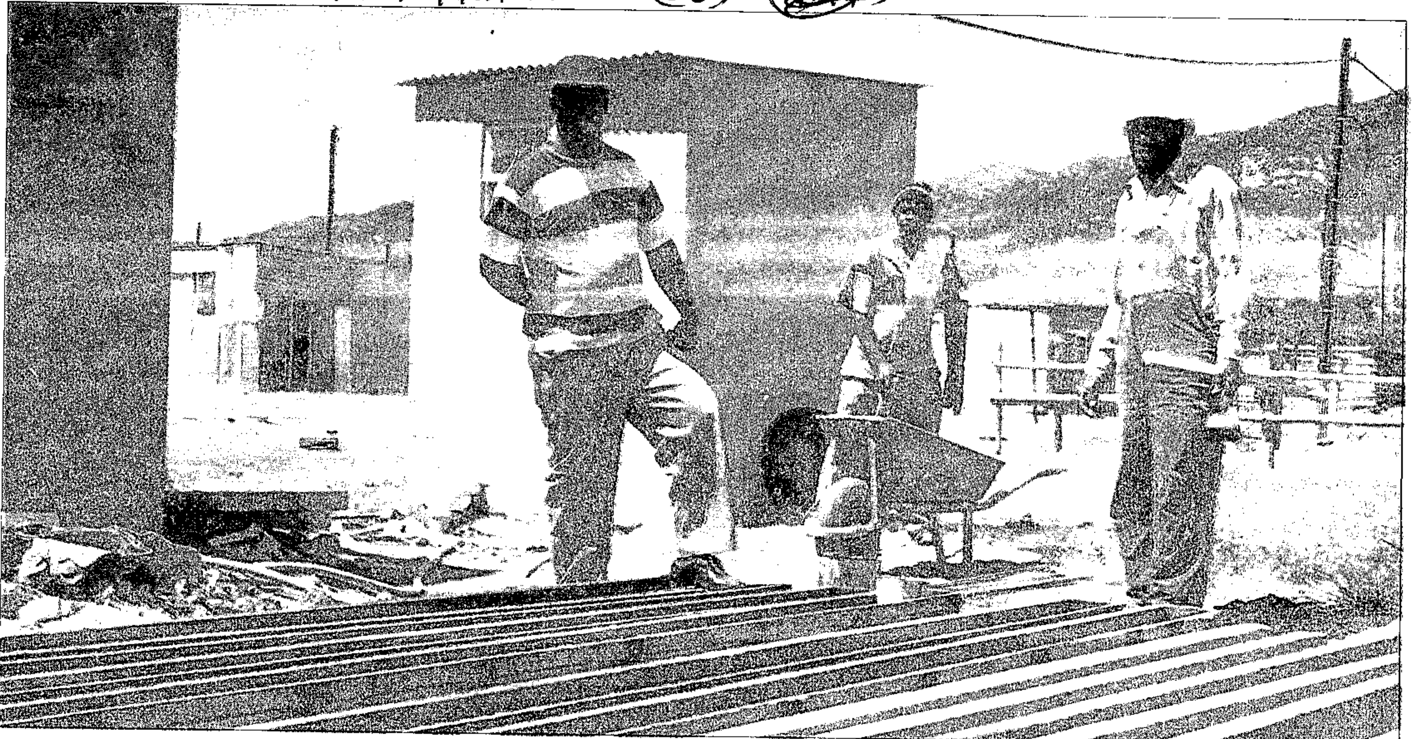
New start: Masiphumelele residents who can afford something better than a wooden shack are being helped by developers Communicare to build brick homes
