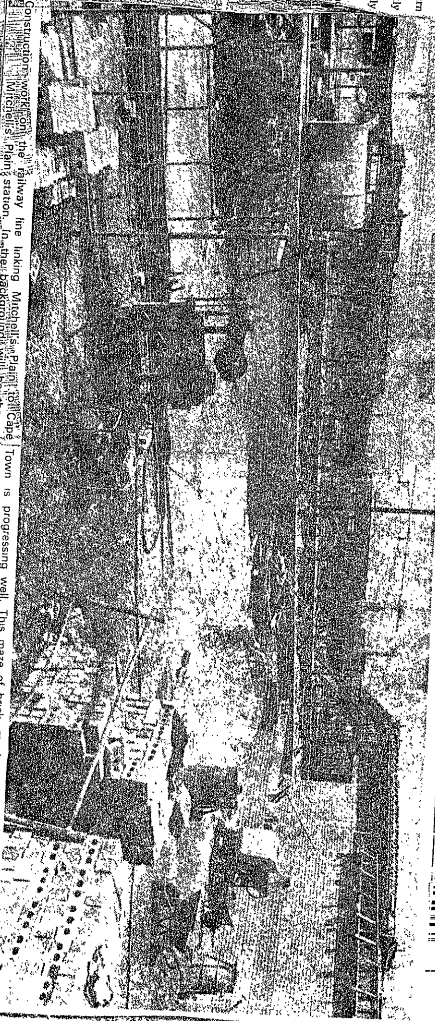
Construction work on the railway line linking Mitchell's Plain to Cape Town is progressing well. This maze of brick, mortar and steel will soon be turned into the Mitchell's Plain station. In the background will be the multi-million rand shopping complex of O K Bazars, Pick 'n Pay and Woolworths.
