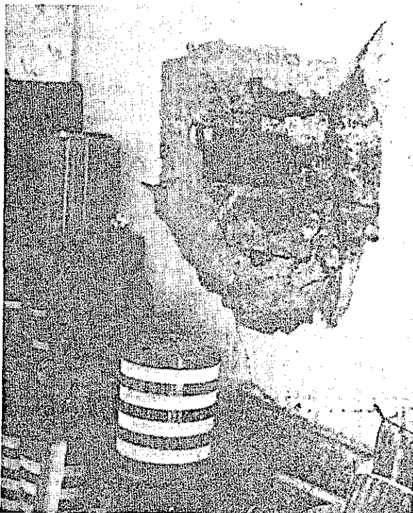
Police in Zimbabwe suspect a rocket-propelled grenade caused this damage to a house in Harare early yesterday. Police believe the grenade overshot its intended target, a neighbouring house occupied by the African National Congress.
