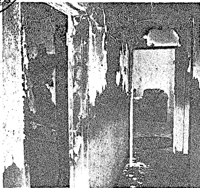
FIRE BOMB: The damaged passage of the Khan home where a petrol bomb was thrown into the room on the left.
