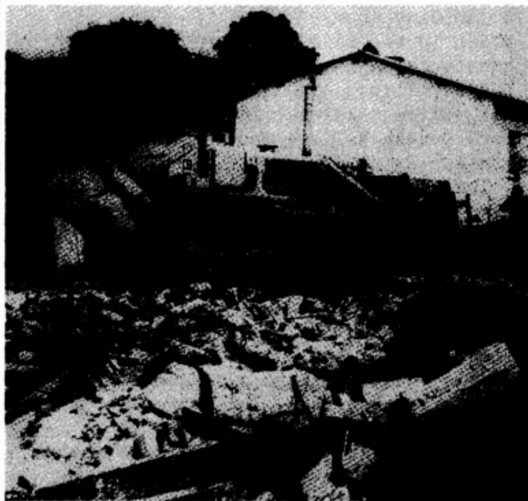
Bulldozer clears rubble from a house in the way of the new bypass road
